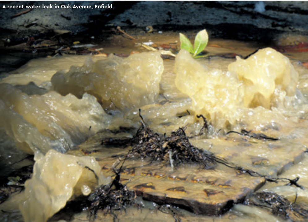
A recent water leak in Oak Avenue, Enfield
